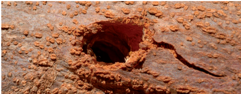
Damage caused by larvae. Entry/emergence hole with frass and wood dust 15
